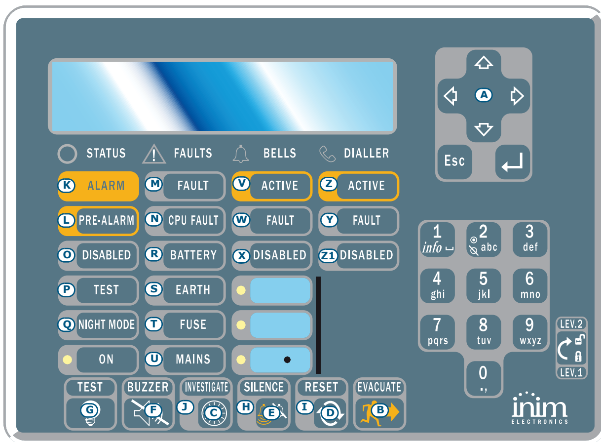
Figure 9 - Front view of the repeater panel
